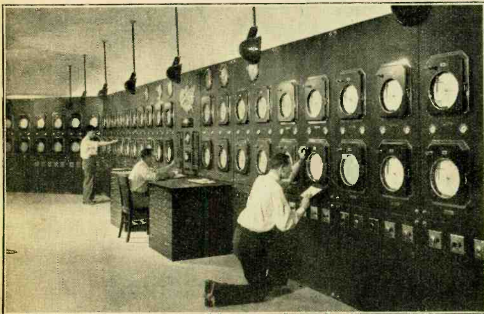
RADIO CITY, NEW YORK, is equipped with this special Air Controlling Plant, whereby the ventilation of each studio can be checked at any moment and changed to suit requirements. There are 64 dials. It is stated that four generators in the basement can produce "900 tons of refrigeration in 24 hours."
